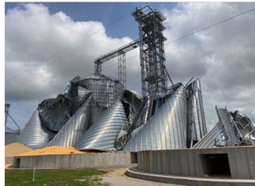
Grain bins destroyed by the derecho in Luther, Iowa. (photo by Justin Glisan)
