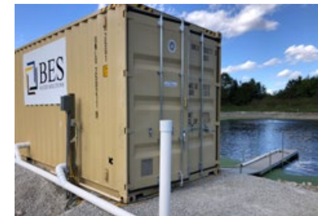
BES Water Solutions moving-bed bioreactor.
