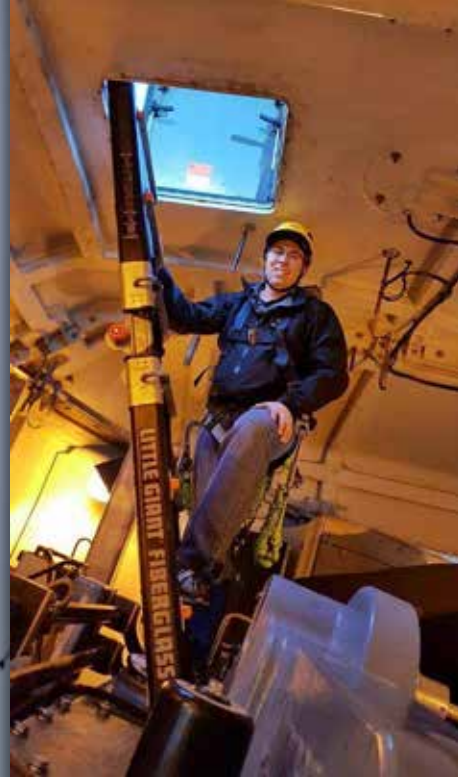
Corey Markfort inside the nacelle of the Clipper 2.5 MW wind turbine at Kirkwood Community College in Cedar Rapids, Iowa. The nacelle is located on top of the tower and contains the generator which connects to the hub of the spinning blades of the turbine.
