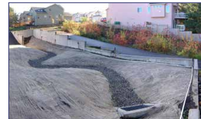
Bioswales are landscape elements designed to concentrate or remove debris and pollution from surface water runoff. This bioswale is under construction.
